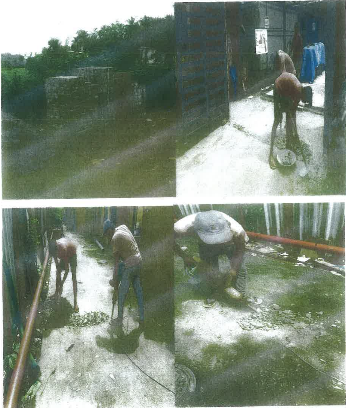
Removal of PCC for replacing with pavers on the Service road to kitchen.
